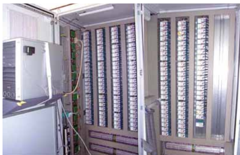
Fig. 6: The inside of the switch cabinet in the measuring technology and control room with more than 160 DC measurement amplifiers and the computer containing A/D converters
